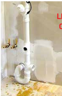
Waste Line coming Through "Cabinet Wall"
