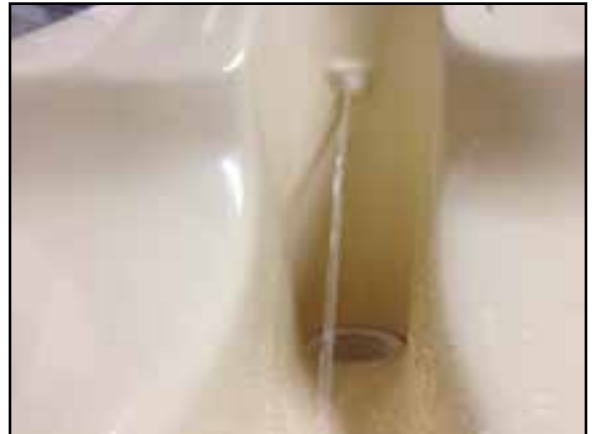
Connector Nozzle Draining into Base Where Waste/Water drains Into Waste Line ( Over 4" Air Gap)
