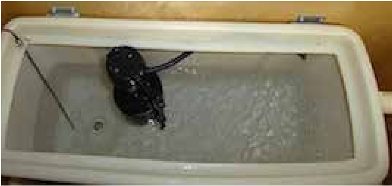
FLUID MASTER 400 FILL FLOAT VALVE INSIDE WATER TANK
