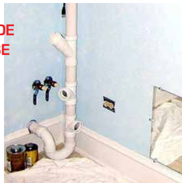
Waste Line coming Through "Head Wall"
