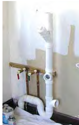
Sewer coming thru "Thru Floor"
