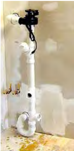
Sewer coming thru "Cabinet Wall"
