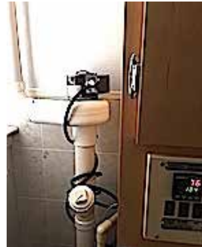
Odor Control Fan shown here going up into the ceiling
