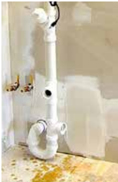
Waste Line coming Through "Cabinet Wall"
